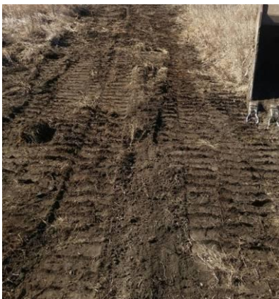
Photo #17 Reclamation of the area in proximity of Cote 2 from dewatering activities.
