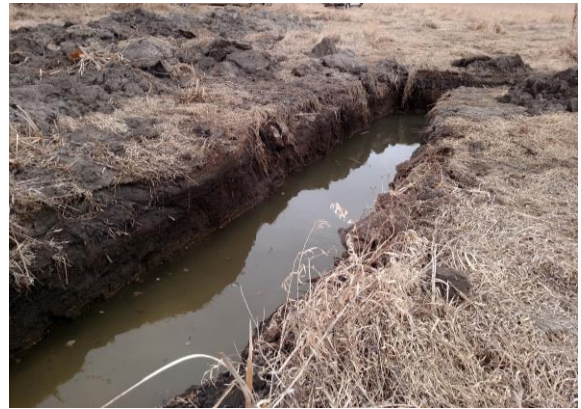
Photo #16 View of impacts from dewatering activities at Cote 2.
